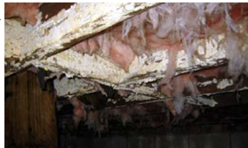
Wood-decaying fungi. damage
