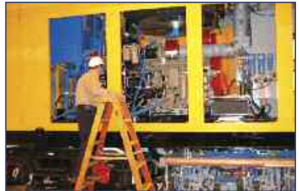
An HTT worker inspects one of the company’s rail grinding machines as it is being built.
