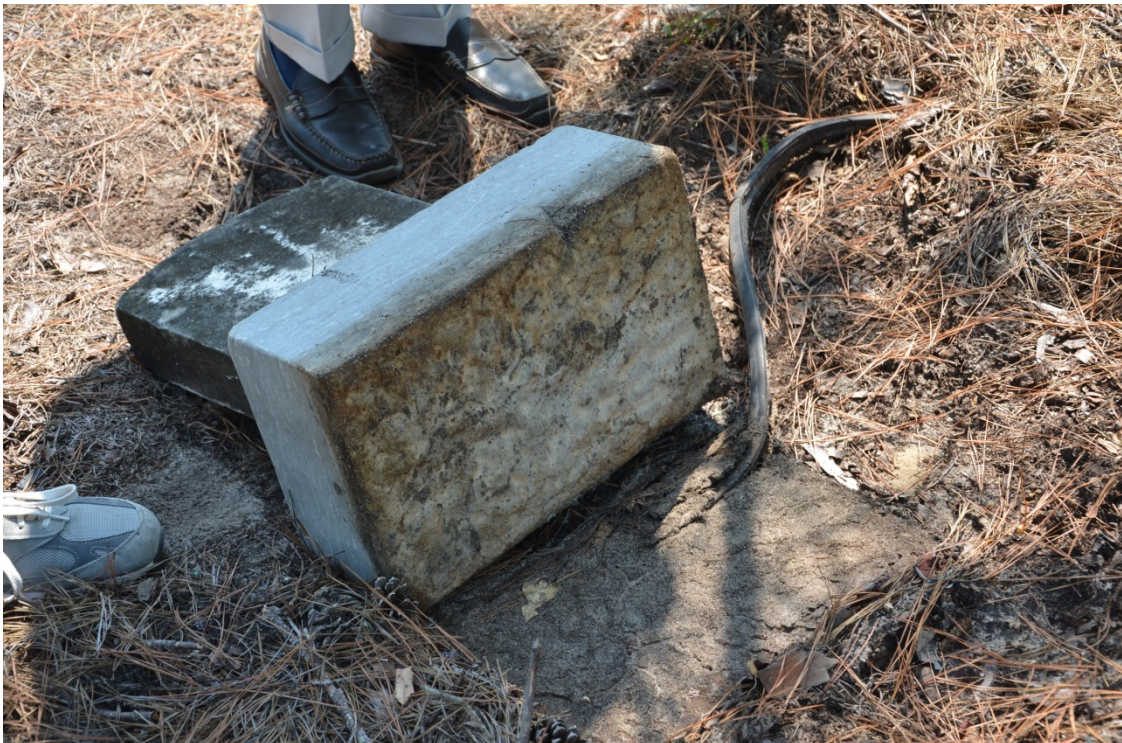
Stone moved showing rubber gasket running under the stone.
