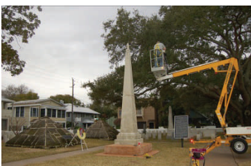
The additional work made use of a small, lightweight lift that could be pushed by hand up to the Dade Monument and not damage the sidewalk.
