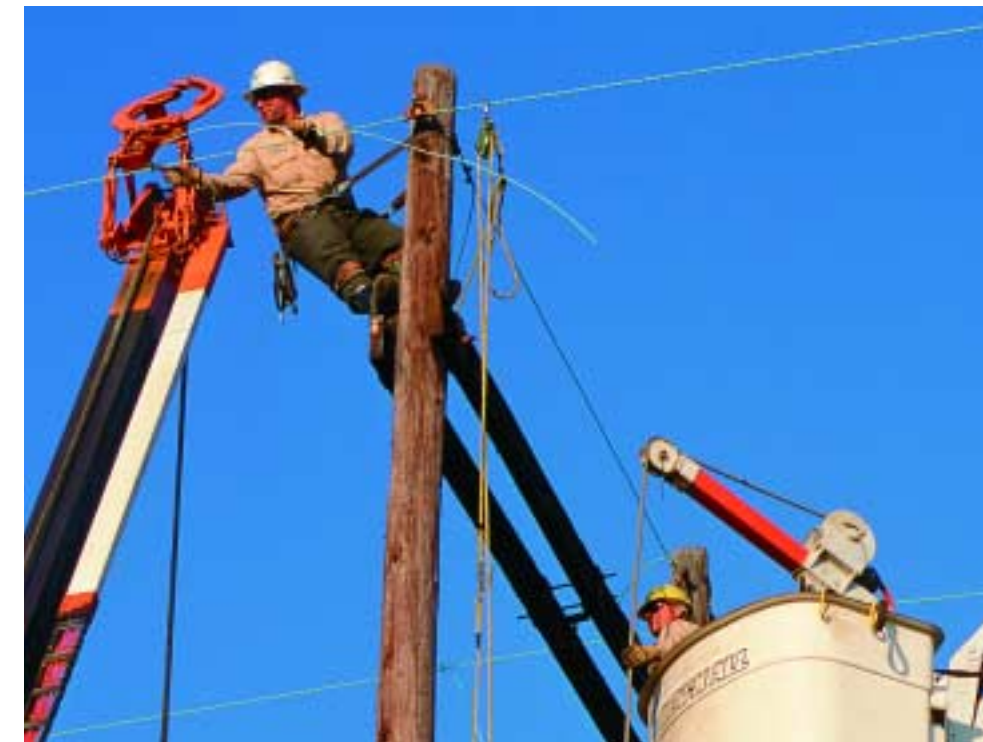
Routine maintenance helps maintain high reliability. Santee Cooper line crew performs work on a transmission line near Overton.
