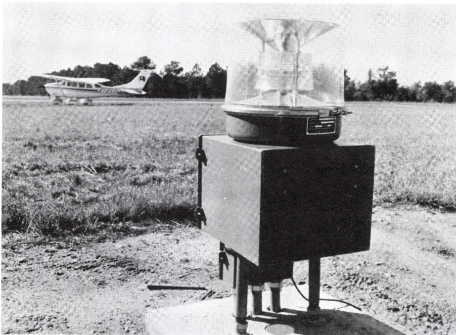
Runway End Identifier Lights (REILS) have been installed at Aiken airport. The strobe lights were funded by a grant from the S.C. Aeronautics Commission. (Aeronautics Commission photo)
