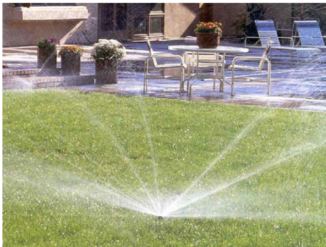
Figure 5. A stream rotor in operation. (Courtesy Hunter Industries)
