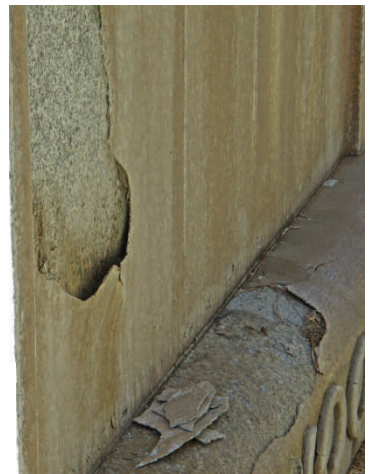
Here the deposits are causing spalling of a granite monument.
