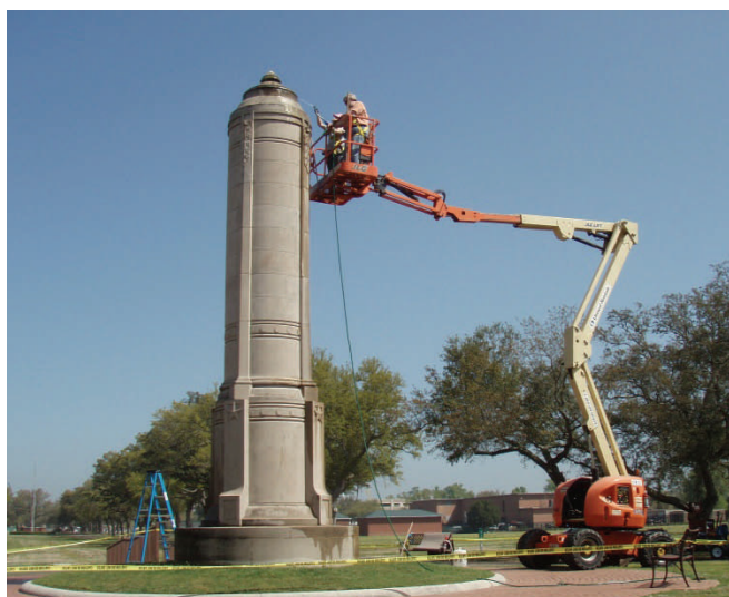
Beginning at the bottom and working up, the Chicora team completely cleaned the monument using D/2.
