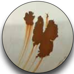
Corrosion due to poor maintenance is a common source of AST failures.
