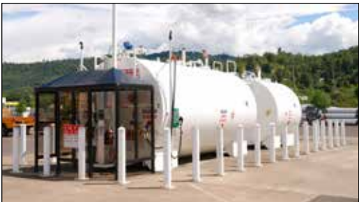
The photograph above shows ASTs with adequate barriers to prevent vehicle collisions.
