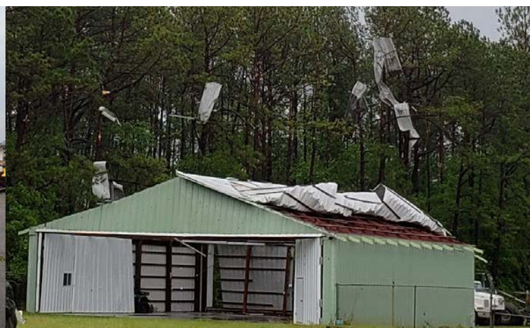
The roof was ripped off the airplane hangar, and debris was stuck in the trees.
