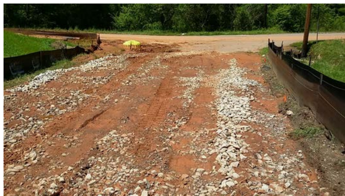
No geotextile fabric was used. Rutting has occurred, and stone is being incorporated into soil below. Photo by Scottie Ferguson, Pickens County Stormwater.
