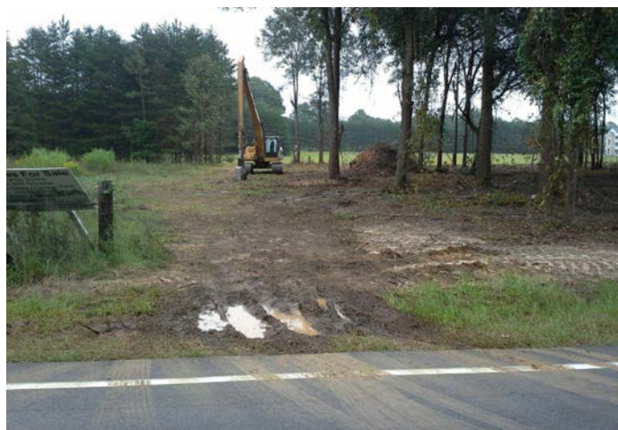
No stabilized entrance. Sediment is tracked onto the roadway and rutting has occurred. Photo by Dan Geddings, Sumter County Stormwater.
