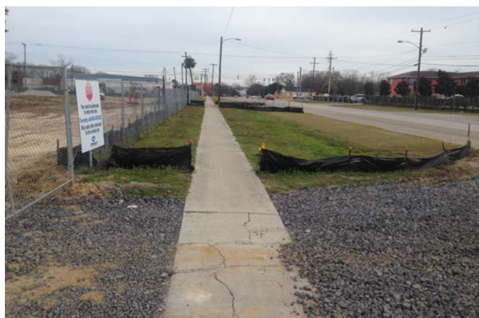
A properly installed construction entrance keeps the road clear of debris and sediment. Photo by Chuck Jarman, Clemson Extension.
