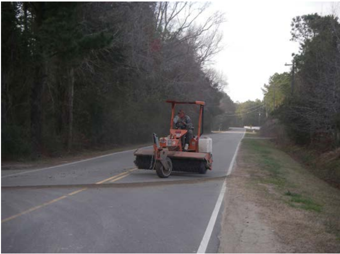
Sediment that was tracked on the roadway is being swept up to keep the roadway clear. Photo by Chuck Jarman, Clemson Extension.
