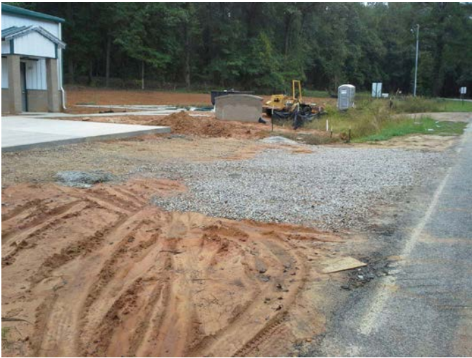
Stabilized entrance needs to be made both longer and wider and tapered out towards road. Photo by Dan Geddings, Sumter County Stormwater.
