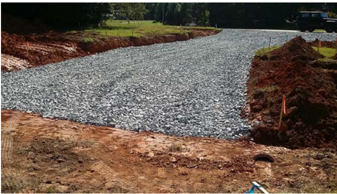
Stabilized entrance with sufficient width and length and is tapered out. Photo by Scottie Ferguson, Pickens County Stormwater.
