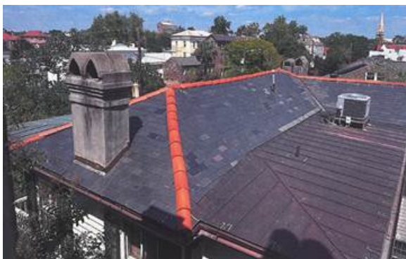
After photograph of the repaired terracotta hip caps and slate roof and replacement copper roof.
