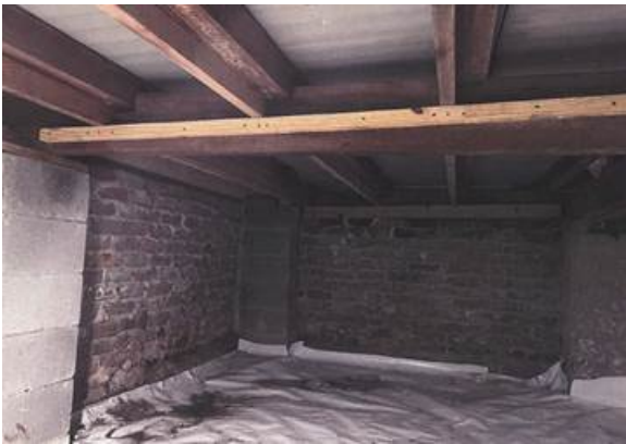
After photograph of the crawlspace, showing sistered joists and historic joists supporting the residence.
