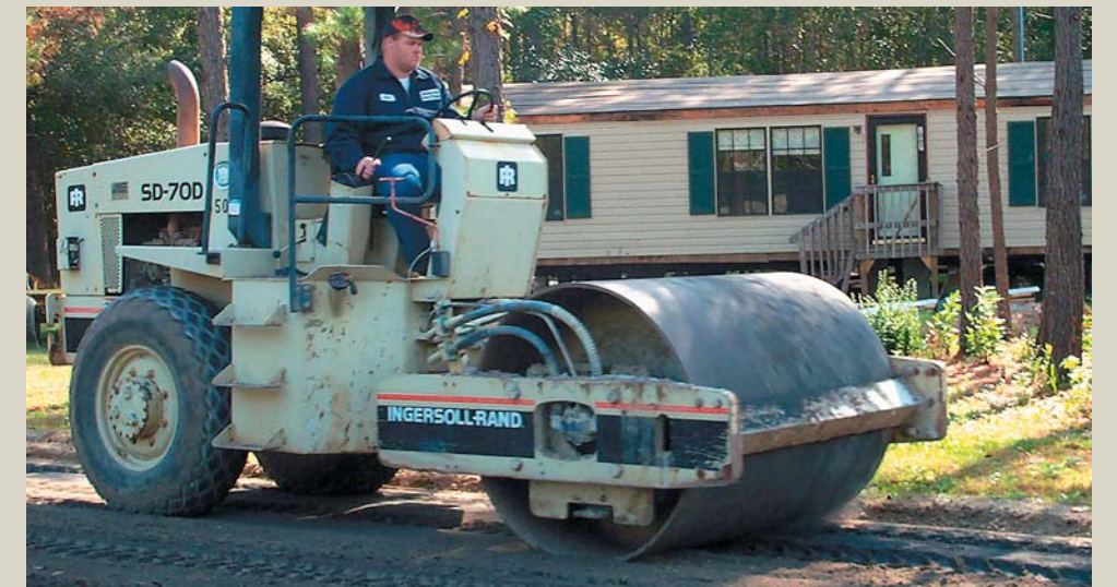
Vibrating roller is used to compact the road prior to the final spray of Earthbind emulsion.
