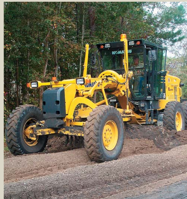
Tobacco Road, near St. Stephen, S.C. is being graded and prepared for application of fly ash and sand.
