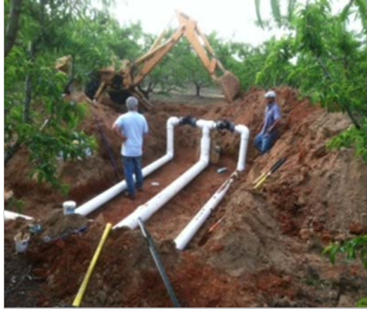
David Lankford, left, with EarthTec Solutions oversees the installation of a splitter valve to regulate irrigation in the test orchard located on JW Yonce and Son farm near Johnston.
