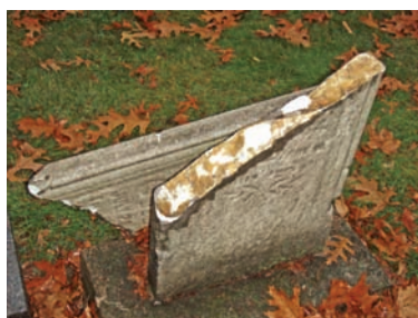
A typical “simple” epoxy repair that was doomed to failure. This inappropriate repair will make a correct repair more time consuming — and costly.
