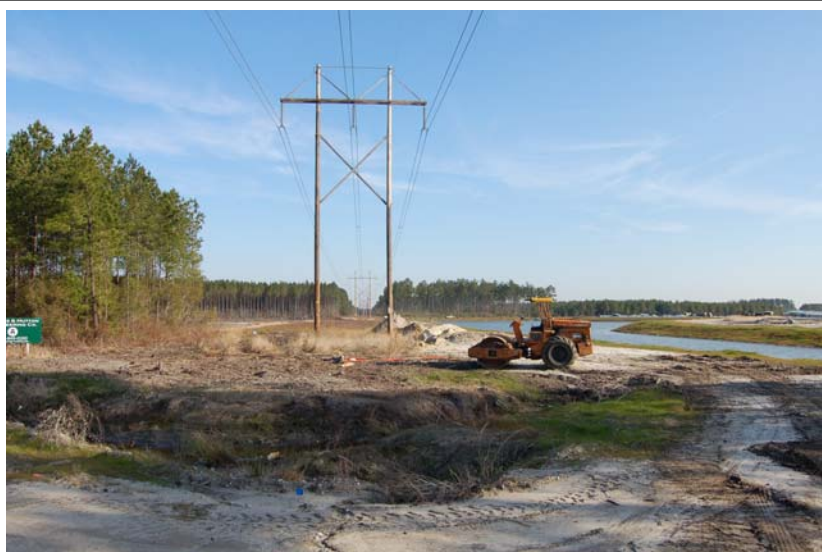
Figure 4. Project corridor through a construction area (parallel to the existing transmission line).
