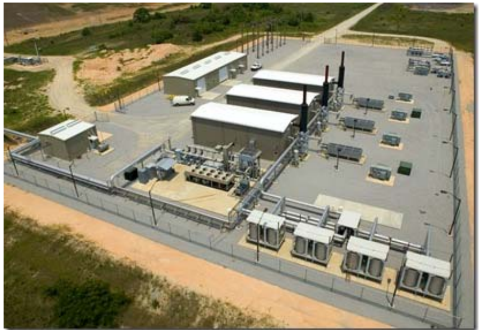
This Santee Cooper electricity generating station in Lee County uses biogas extracted from an Allied Waste landfill. (Photo/Jim Huff, Santee Cooper)
