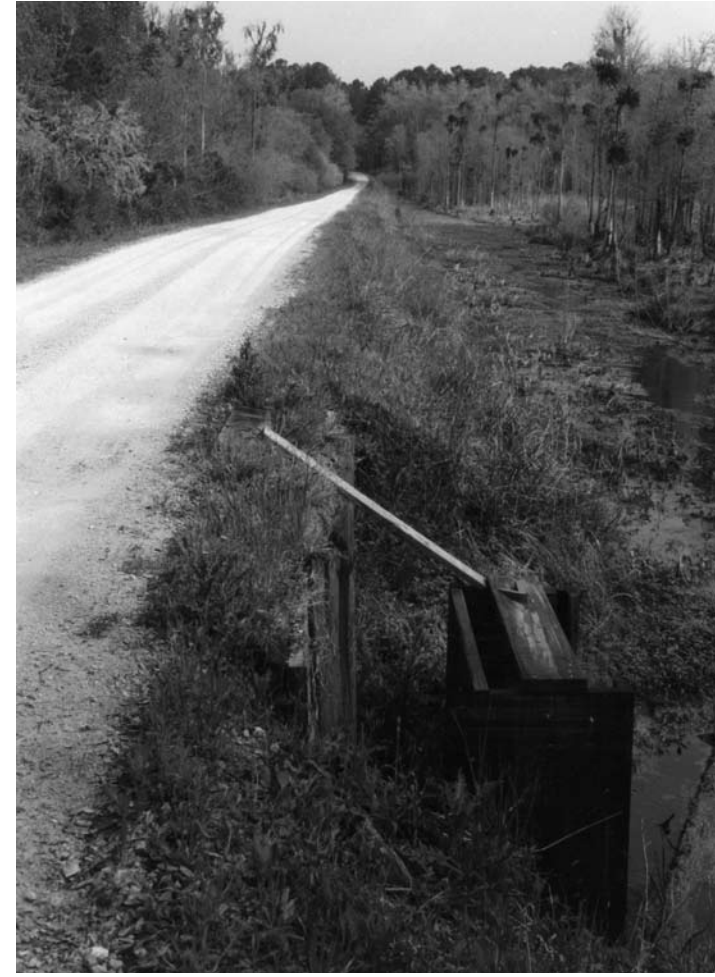
The Driving Trail crosses several causeways, many built originally by inland rice planters and now part of the property's wetlands management system.
