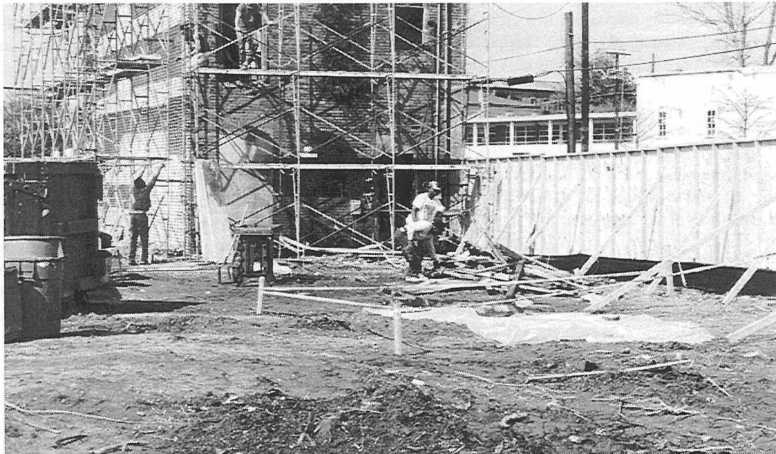
Figure 56. Rehabilitation had already begun on 40 Archdale Street by the time of our excavations. This view also shows the location of Units 1 (background) and 2 (foreground).
