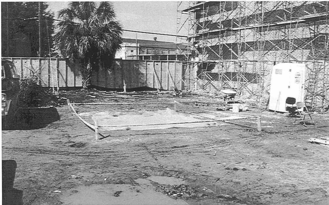
Figure 63. Area of Unit 3, south of 40 Archdale Street, behind 38 Archdale. View to the northwest.
