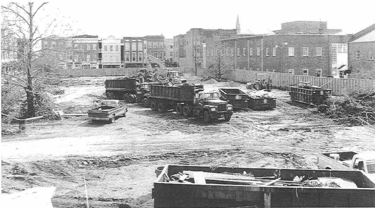
Figure 55. Eastern half of the project block showing construction activity and the removal of the demolished bank building.
